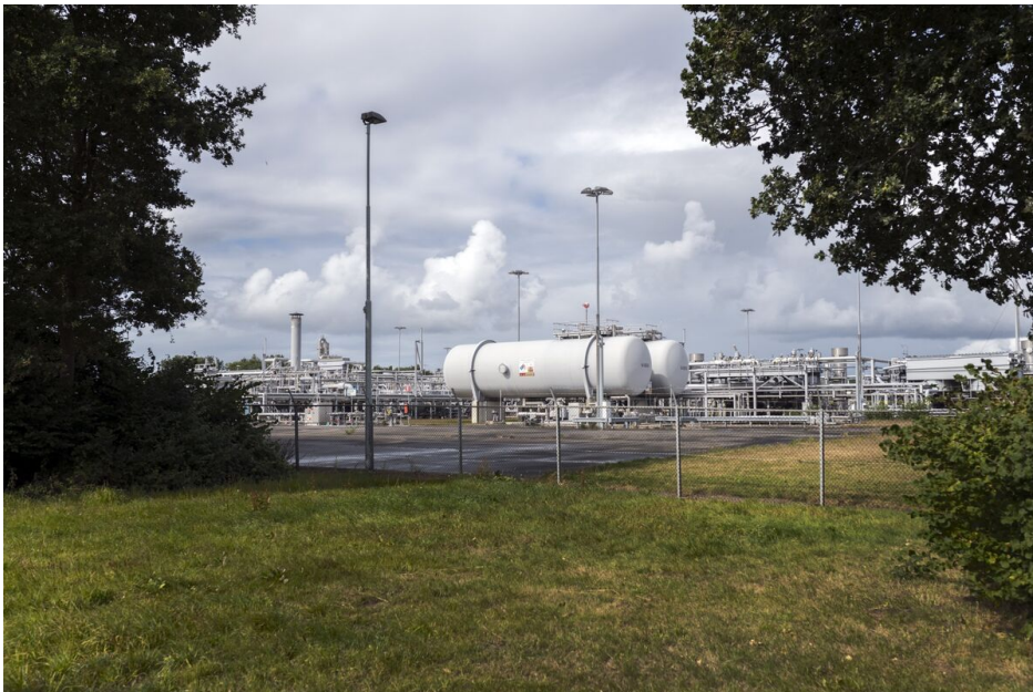
A gas extraction and treatment station in Tusschenklappen, Netherlands. Photographer: Imke Lass/Bloomberg
