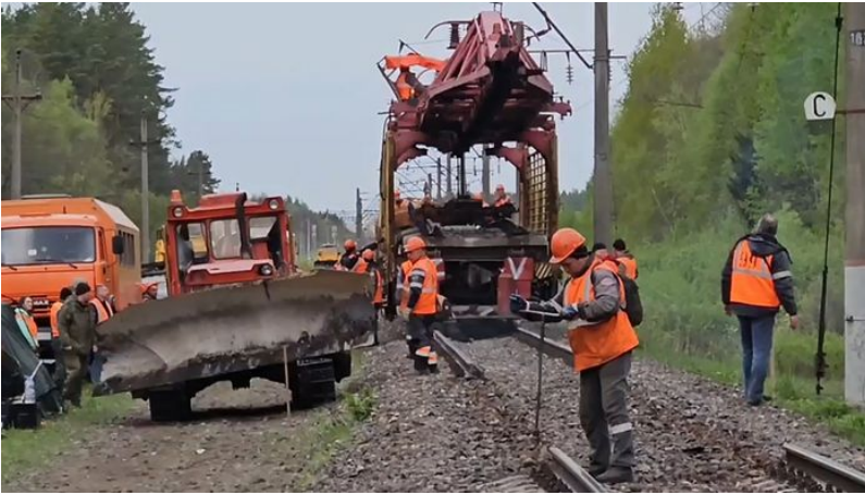
Workers repair a railway track at the site of a blast in Russia's Bryansk region. PHOTO: RZD RUSSIAN RAILWAYS/ZUMA PRESS
